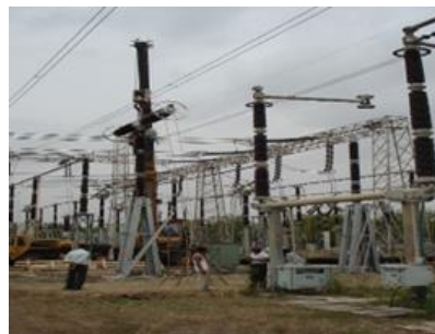
Image – 5 Maintenance personnel working without safety equipment
