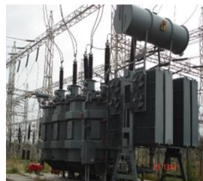
Image – 15 Transformer without Water Sprinkler Fire System
