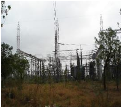
Image – 9 Vegetation growth in switchyard area
