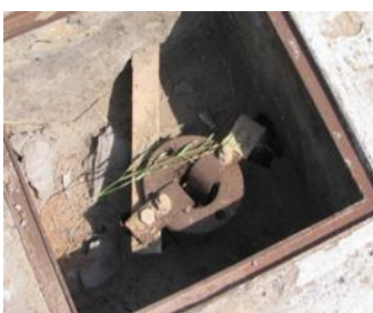
Image – 1 Improper maintenance of earthing pit
