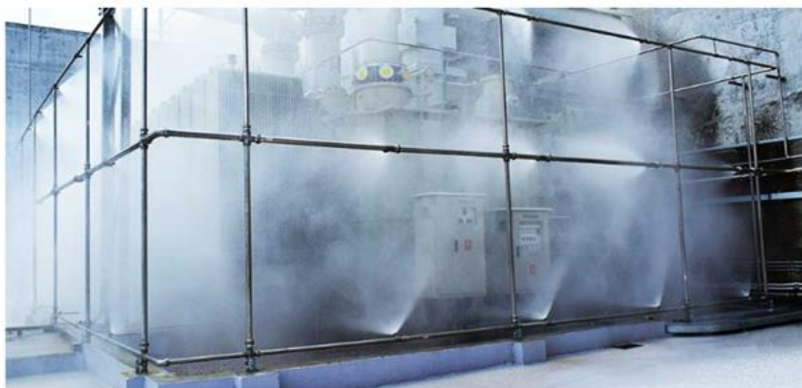
Figure:3 Water Sprinkling System in operation
