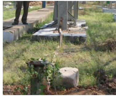
Image – 2 Improper maintenance of earthing pit
