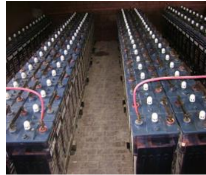
Image – 12 Properly maintained battery room
