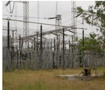
Image – 3 Improper covering of motor pump
