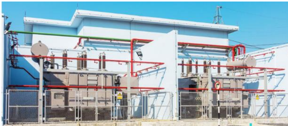
Figure:2 Water Sprinkling System
