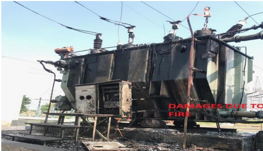
Figure:9 After fire extinguished
