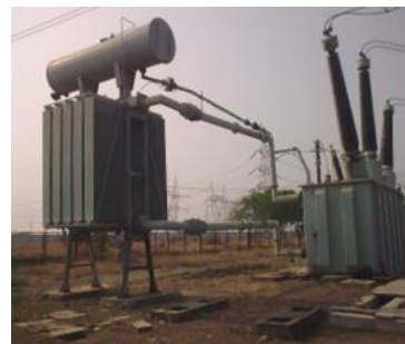
Image – 4 Open earthing pit and cable trench
