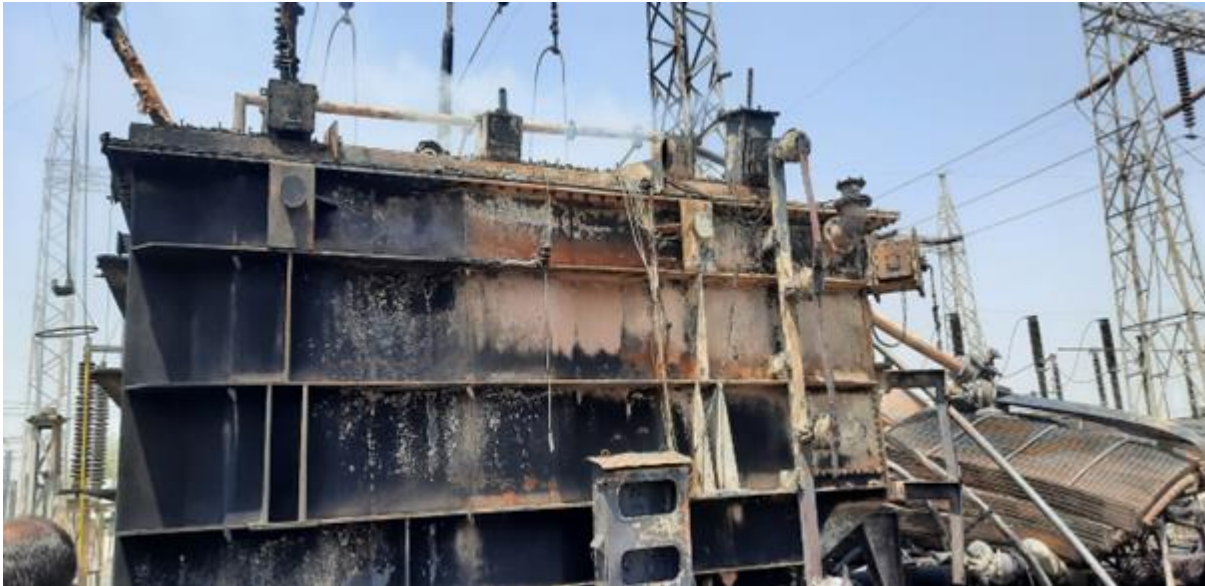
Figure:7 After Fire extinguished
