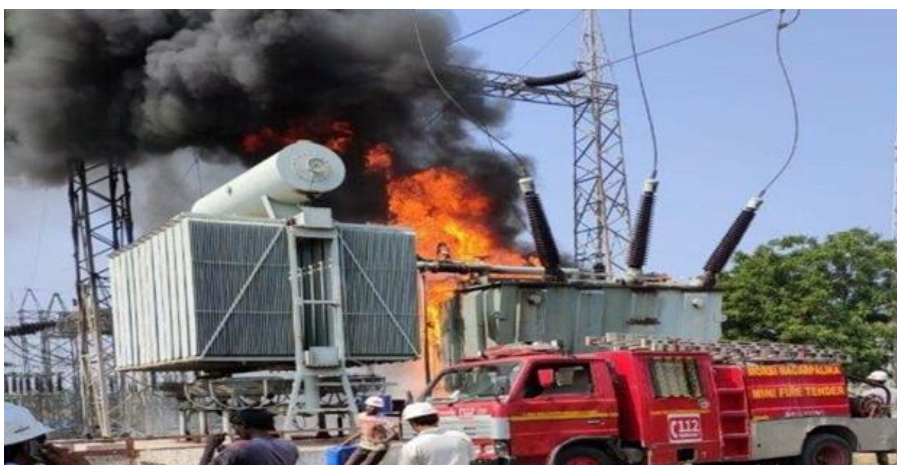
Fig:8 Transformer fire
