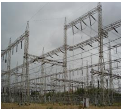
Image – 9 Vegetation growth in switchyard area
