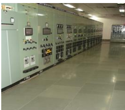
Image – 11 Properly maintained control room
