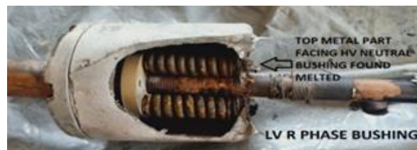
Fig:10 Damaged bushings
