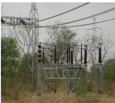
Image – 10 Vegetation growth in switchyard area
