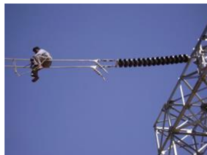
Image – 6 Maintenance personnel working without safety equipment
